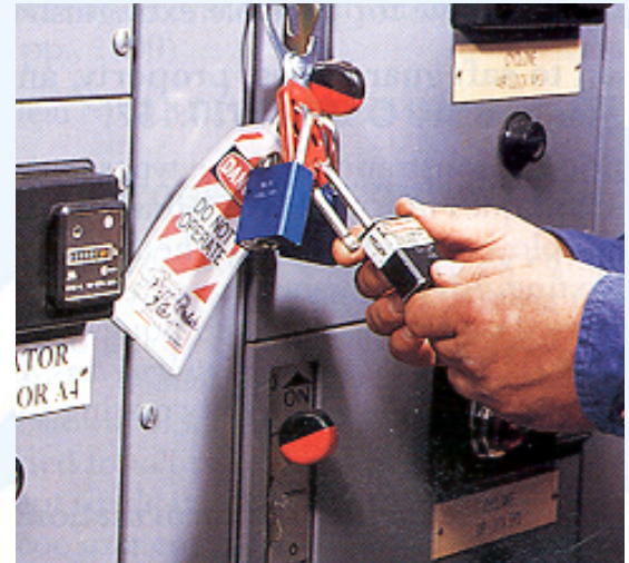
Controls to verify energy isolation
