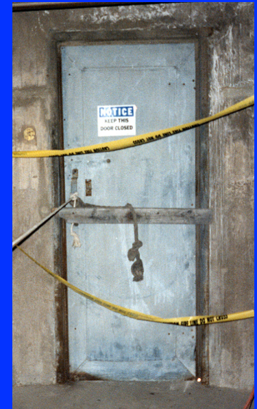
Locked and blocked exit
